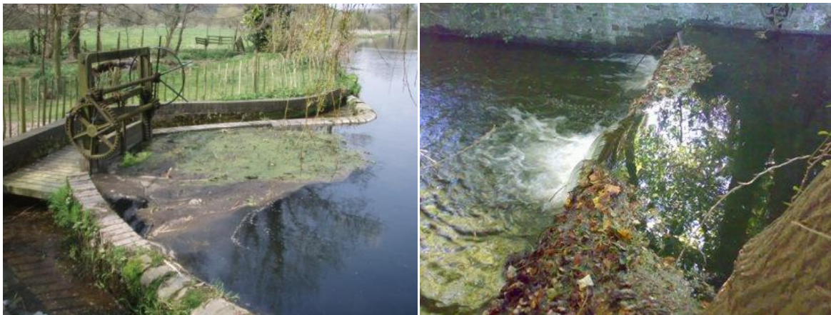
Figure 5.2: Examples of obstructions to fish passage present on the River Chess; river control structure at Sarrattmill House (left) and weir at Chess Falls (right)
